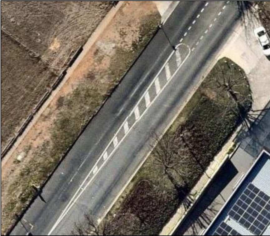
Figure 9 Site access line marking requires modification – design drawing to be prepared
