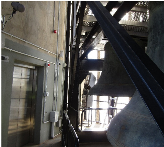
Figure 3.34 View within the Bell Chamber. Note the wall-mounted microphone and conduits. (Source: GML, July–August 2019)
