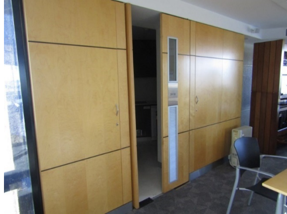
Figure 3.39 Access doors into kitchen located within the service shaft at the Chimes Level. (Source: GML, July–August 2019)
