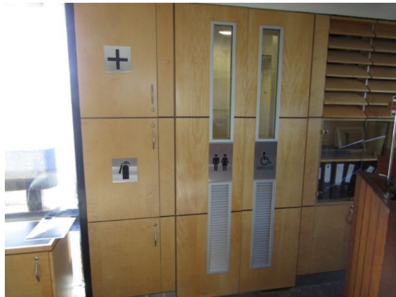
Figure 3.31 Access doors into the toilet and shower area at the Clavier Level. (Source: GML, July–August 2019)
