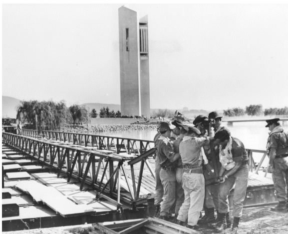
Figure 2.21 Army engineers from Holsworthy, NSW, dismantling the floating bridge, c1970. (Source: ACT Heritage Library, Ref. 005398)
