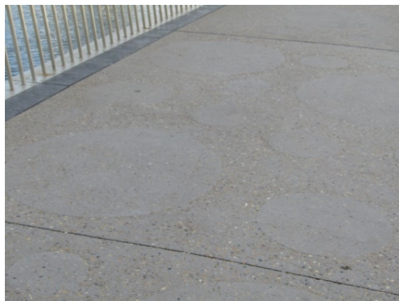
Figure 3.13 Detail of the surface of the bridge, which is exposed aggregate concrete with circles incorporated into the finish. (Source: GML, July–August 2019)
