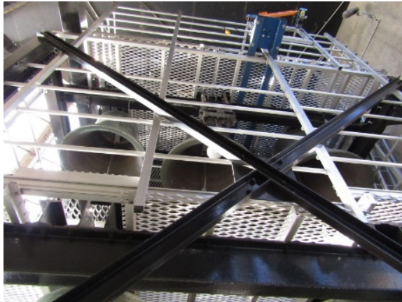
Figure 3.32 View of the Bell Chamber showing the steel frame and mesh gangway system. (Source: GML, July–August 2019)
