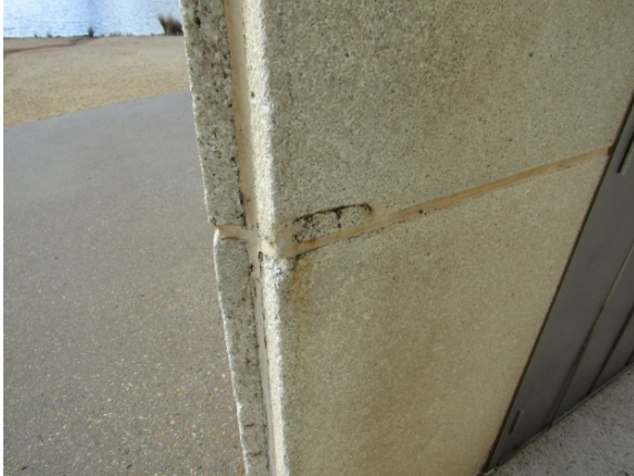
Figure 3.24 Detail of cracking and discolouration on inner façade of shaft. (Source: GML, July–August 2019)
