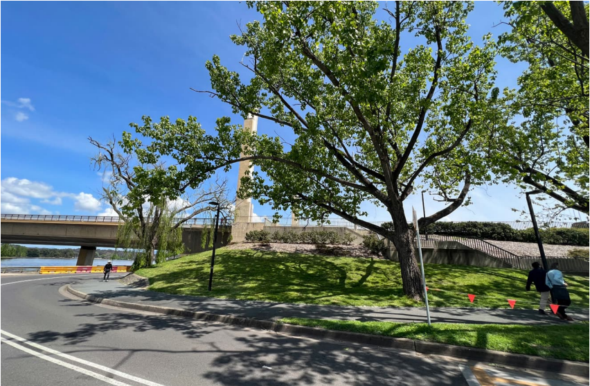
Figure 78: NE Pylon and stair from across Barrine Drive.
