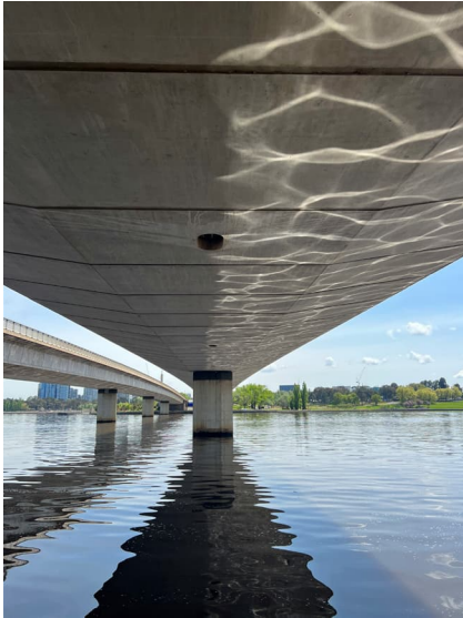
Figure 112: Soffit of southbound bridge showing hole with lighting.
