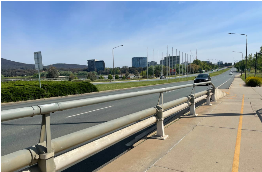
Figure 86: Current barrier termination.
