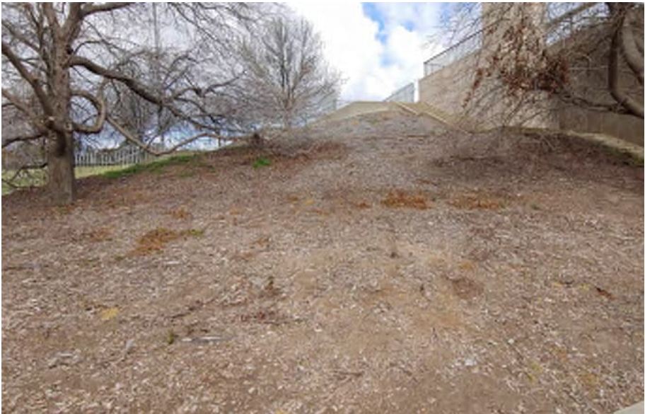
Sloped areas without dense plantings are unsightly and experience erosion
