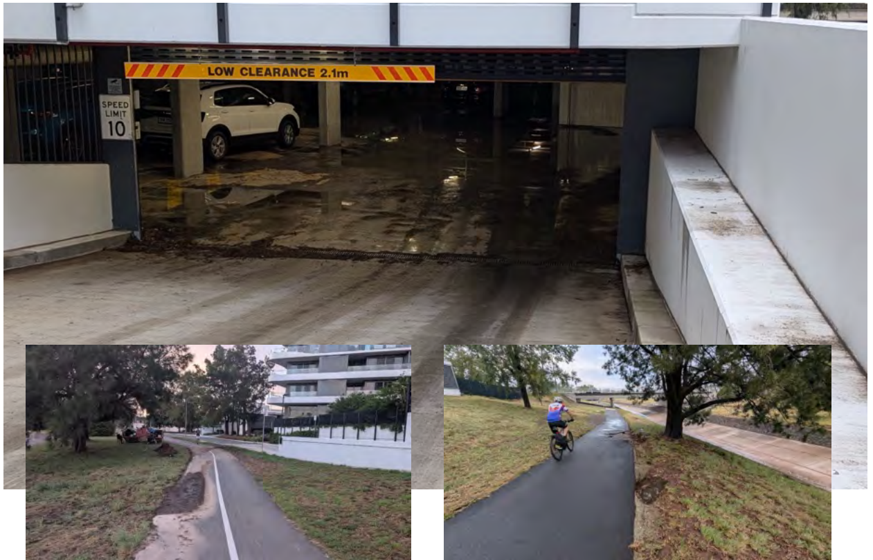
Figure 8 - Feb 2026 Flood damage to building and bicycle path South of Melrose Drive Yarra Glen Intersection
