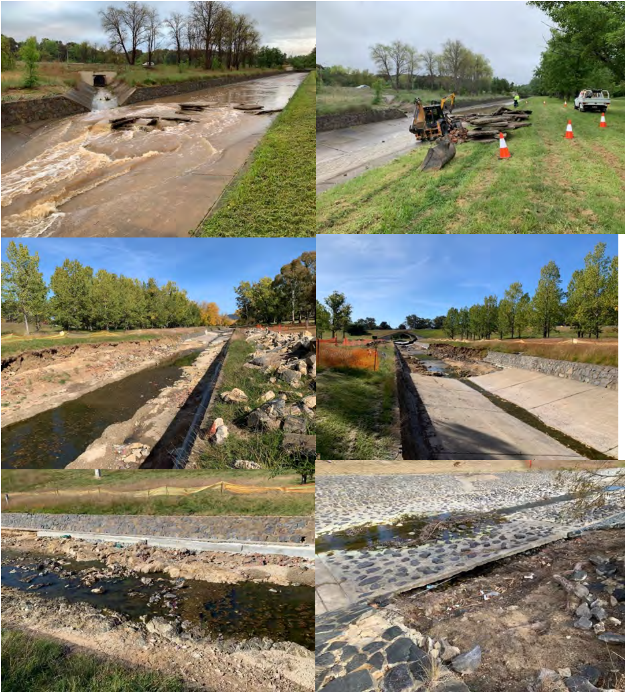
Figure 6 - Recent and current damage to creek lining
