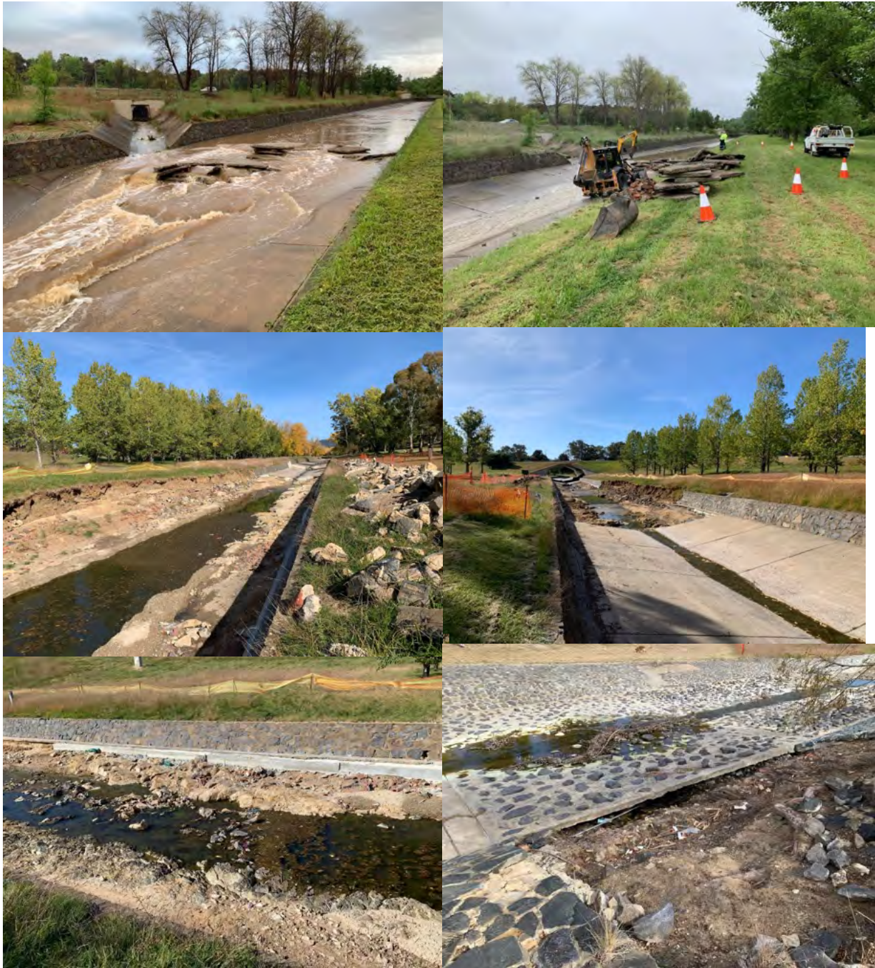
Figure 6 - Recent and current damage to creek lining
