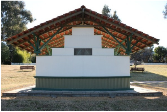
Figure 35: External rear wall of Chapel with glass panel to allow light in to the altar. (Source: GML, 2011)
