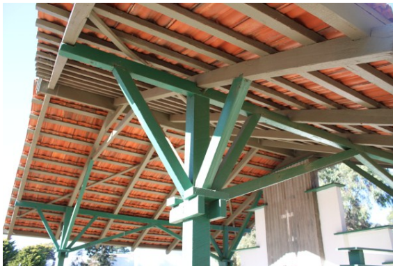
Figure 29: Timber frame construction with hardwood posts and supporting timber arms. (Source: GML, 2011)
