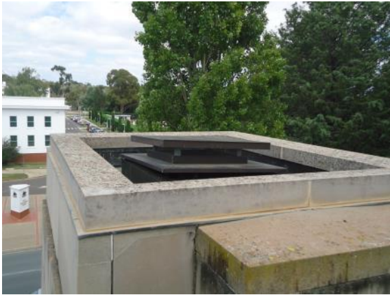
Figure 2.16 View of the top of the memorial and the access hole—the only access route before the construction of the 1996 underground access shown in Figure 2.15. (Source: GML 2013)
