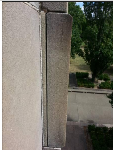
Figure 5.5 Out of plane panel and gap between a thick section of mortar and sandstone panel.
