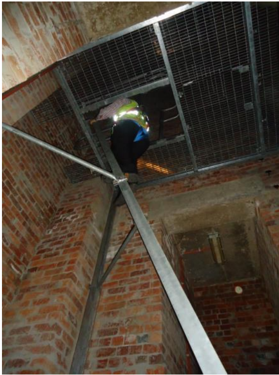
Figure 2.14 Internal view, looking upward, showing brickwork and steel stairs. Note also the large concrete lintel. (Source: GML 2013)
