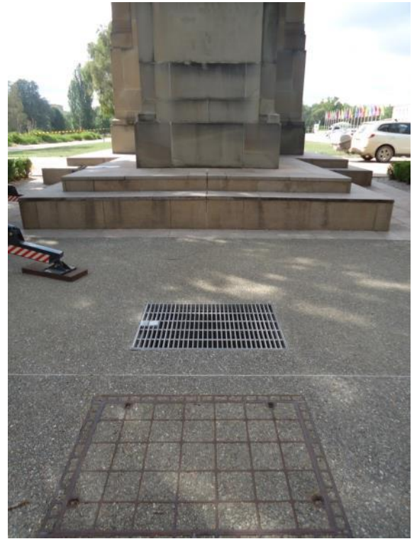
Figure 2.15 Internal access to the memorial is via the grated hatch. (Source: GML 2013)
