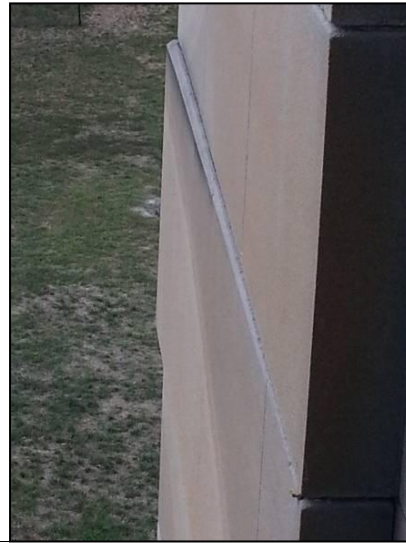
Figure 5.4 Out of plane panel on the northeast façade.
