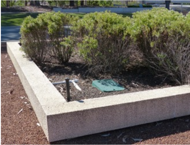
Figure 119. Irrigation infrastructure throughout the beds
