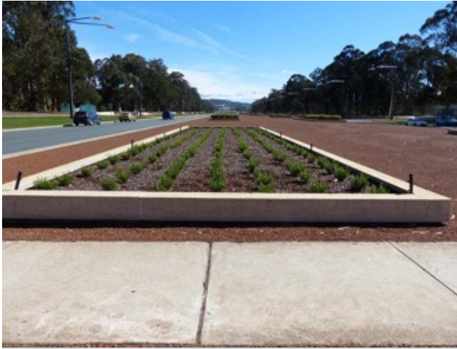
Figure 124. Newly planted Hebe sp. with a linear planting pattern and both sides planted close to the edge
