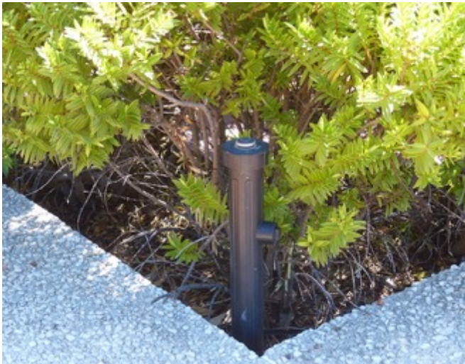
Figure 120. Spray risers blocked by plants
