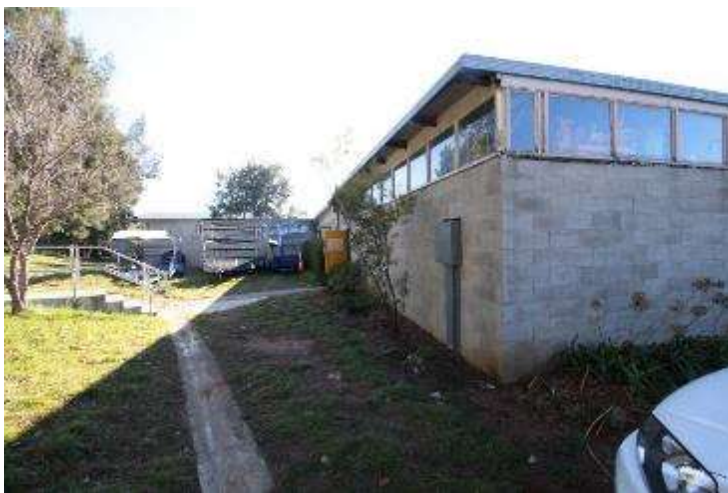
View of front of CRC shed showing existing spoon drain running across corner of site (Fig 12)
